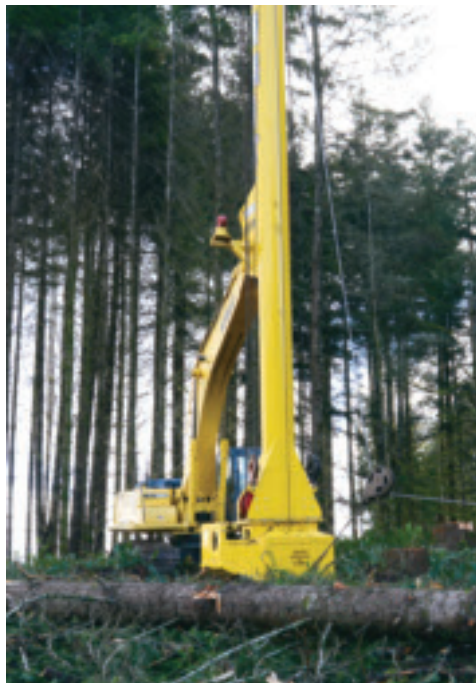
An unmanned excavator equipped with a winch and yarder tower sits at the top of the hill.
