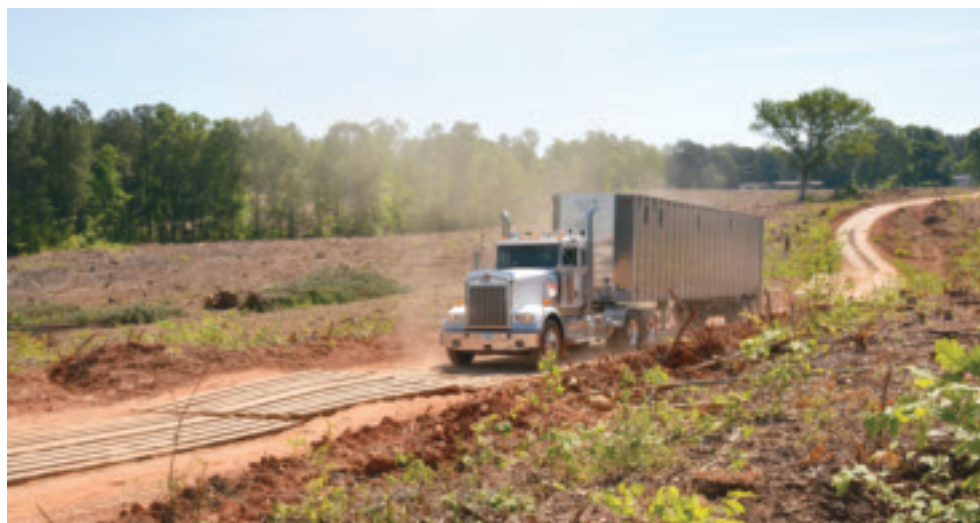
C.K. owns six of his own trucks and trailers. The log trucks won’t get stuck on this well constructed mat road.
